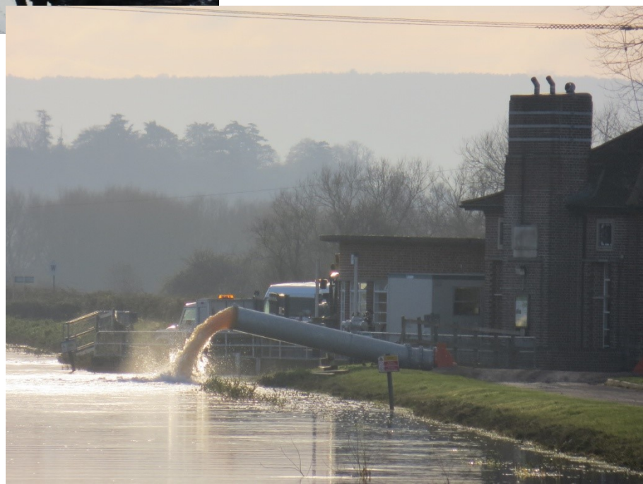
Currymoor pumping station with additional pumps
