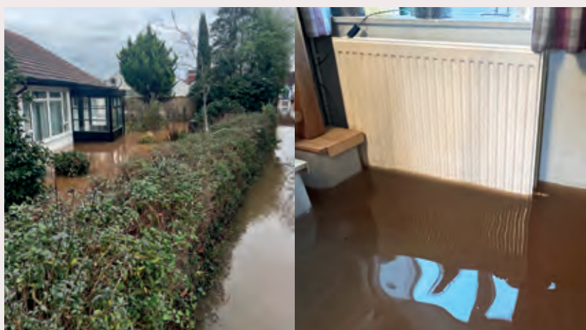
Flooding in Bathpool
